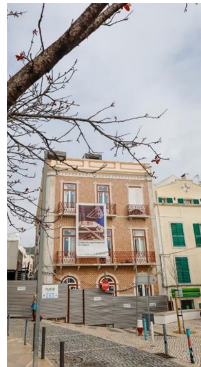
Figure 4 Model of the rehabilitated building (left) and building during rehabilitation, in March 2024 (right). Source: CCC information brochure, 2022 (left), SMM Facebook (right).
